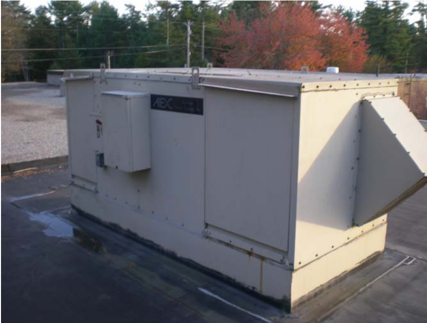
Typical Rooftop Energy Recovery Ventilation Unit (1994 Installation)
