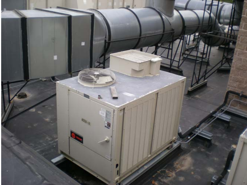
Typical Rooftop Condensing Unit for A/C
