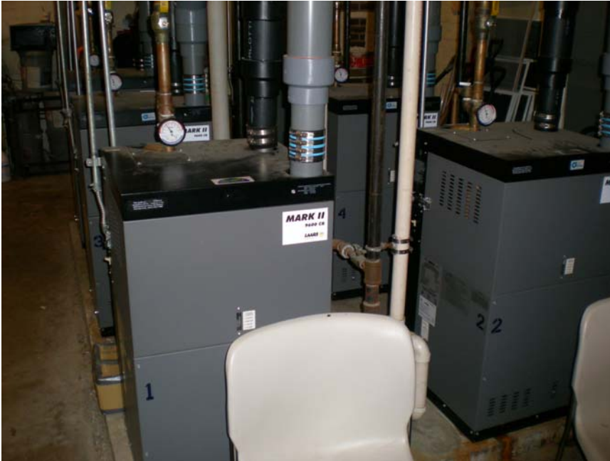
Boiler Plant #2 – Modular Condensing Boilers (2008 Installation)
