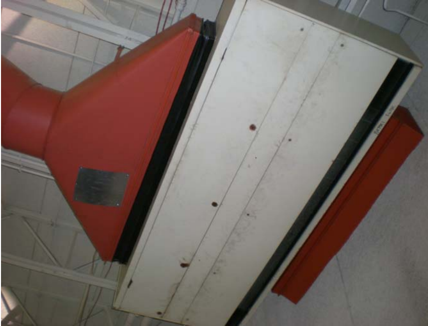
Multi-Purpose Room Unit Ventilator (1979 Installation)
