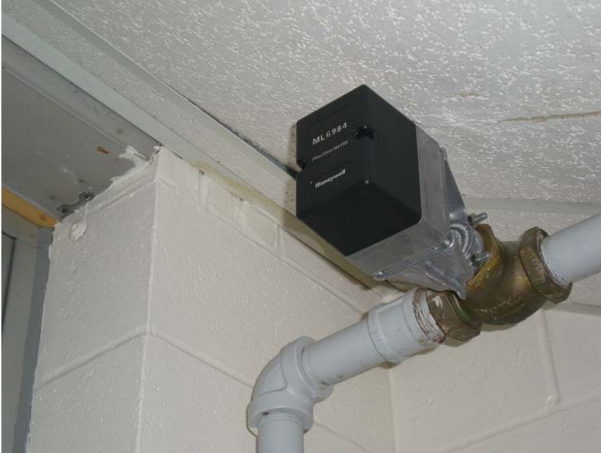
Older vintage heating zone control valve & actuator
