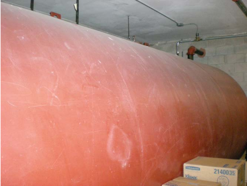
Approx. 5,000-gallon Fire Protection storage tank in shed
