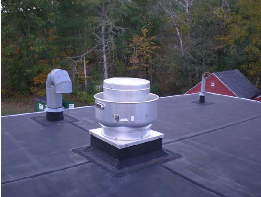
Kitchen Hood Exhaust Fan and Dishwasher Exhaust Fan Discharge
