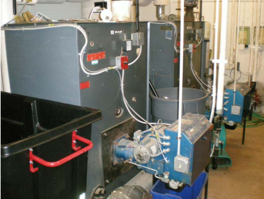
Cast Iron Boilers (1989 Installation)
