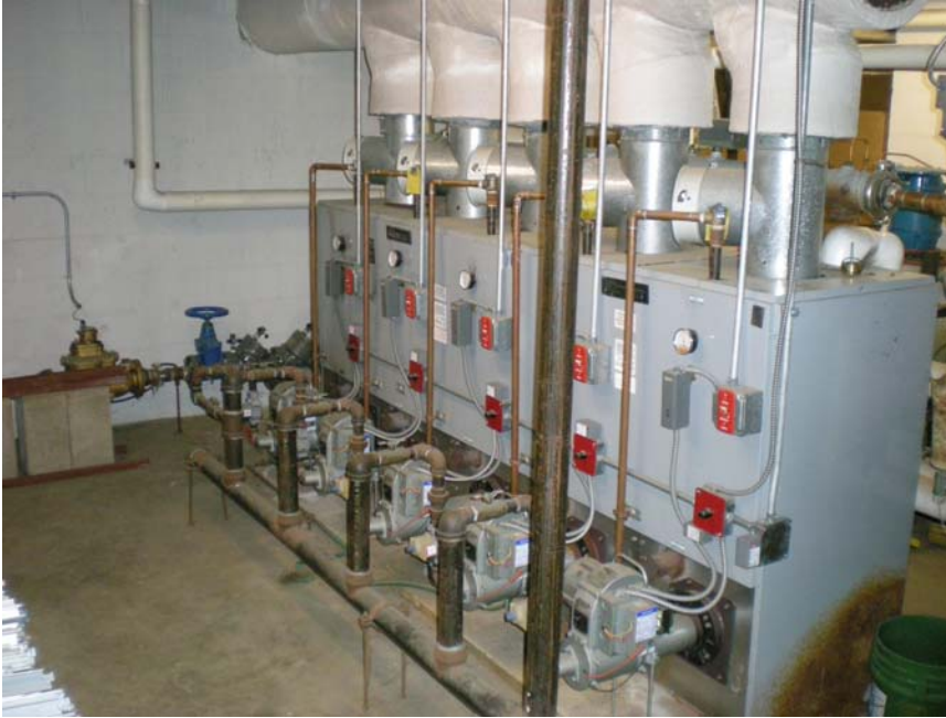
Heating Plant #1 – Modular cast iron boilers (1995 Installation)
